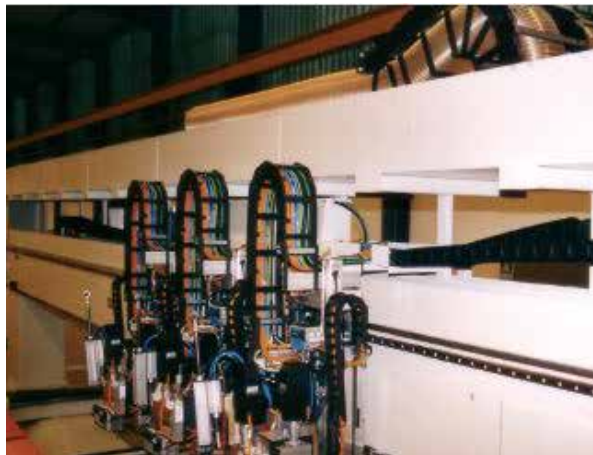
Woodworking machines with e-chains® and chainflex® cables
