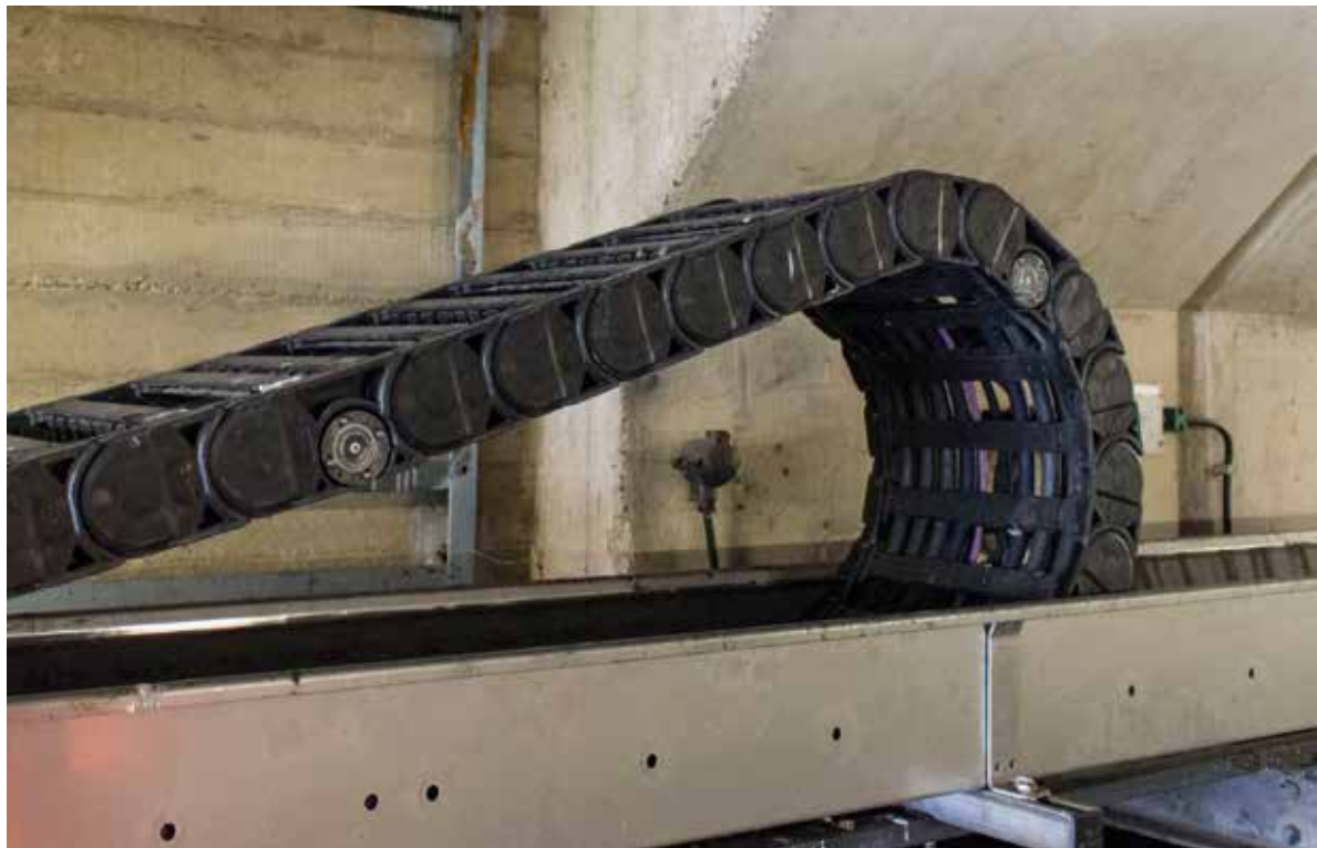
chainflex® Fiber Optic Cable in sea lock
