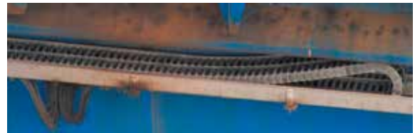
An igus® energy supply system with an approx. length of 85 ft. in a stainless steel trough.
