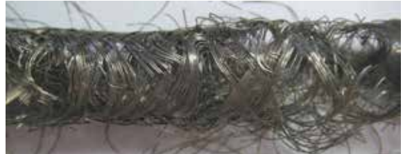
The detail inspection of the shield braid shows distinct damage on the shield wires.
